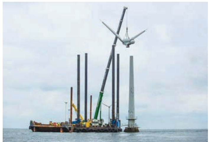
Figure 6. Orsted completed decommissioning of the Vindeby Wind farm in September 2017 after 25 years of service. (Image Credit: MassCEC)
