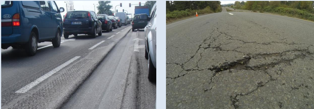
Figure 15. Heat damage to asphalt pavements: Rutting and cracking
