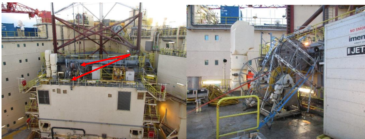
Illustration 7: The photograph on the left shows where the cable reel was positioned for reeling out while the raw water pump was being positioned. The photograph on the right shows the overturned scaffolding.
