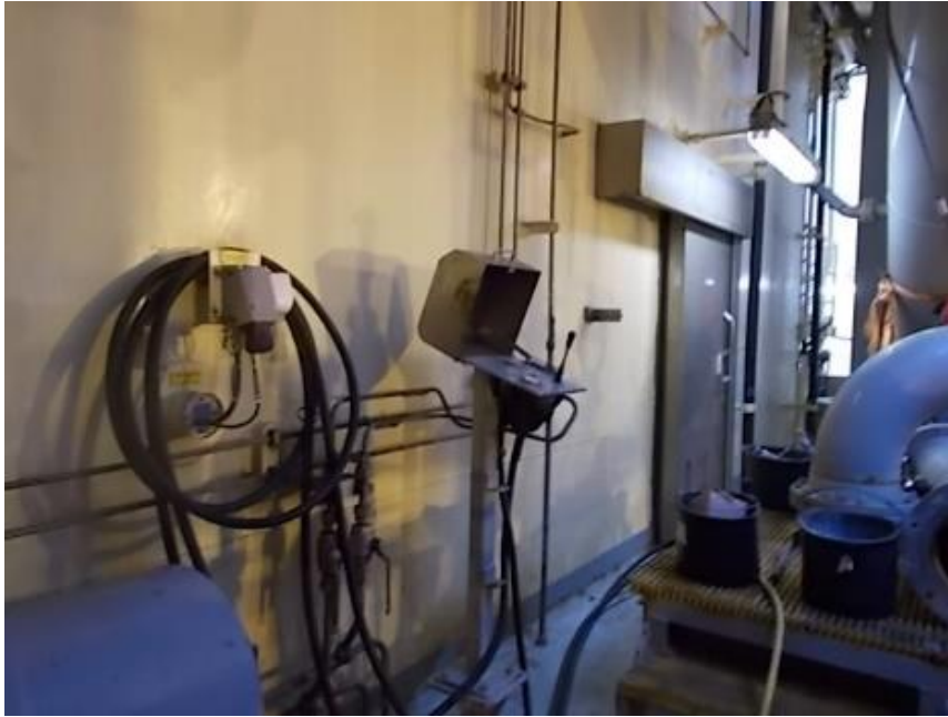
Illustration 14: Operation panel and control valves to operate the relieving system for the raw water pump.
