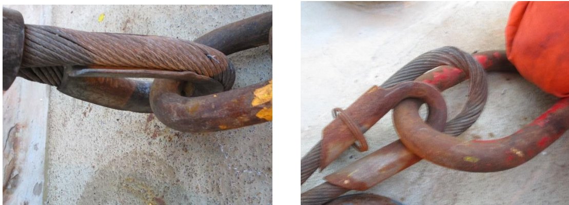
Illustration 13: Damage to the crane pennant used when moving the pump and cable from the deck to the roof of the ventilation housing.
