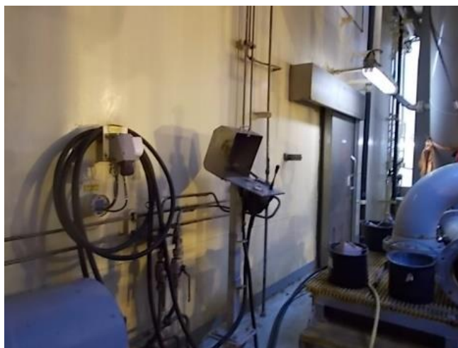
Illustration 12: Operation panel and control valves to operate the relieving system for the raw water pump.
