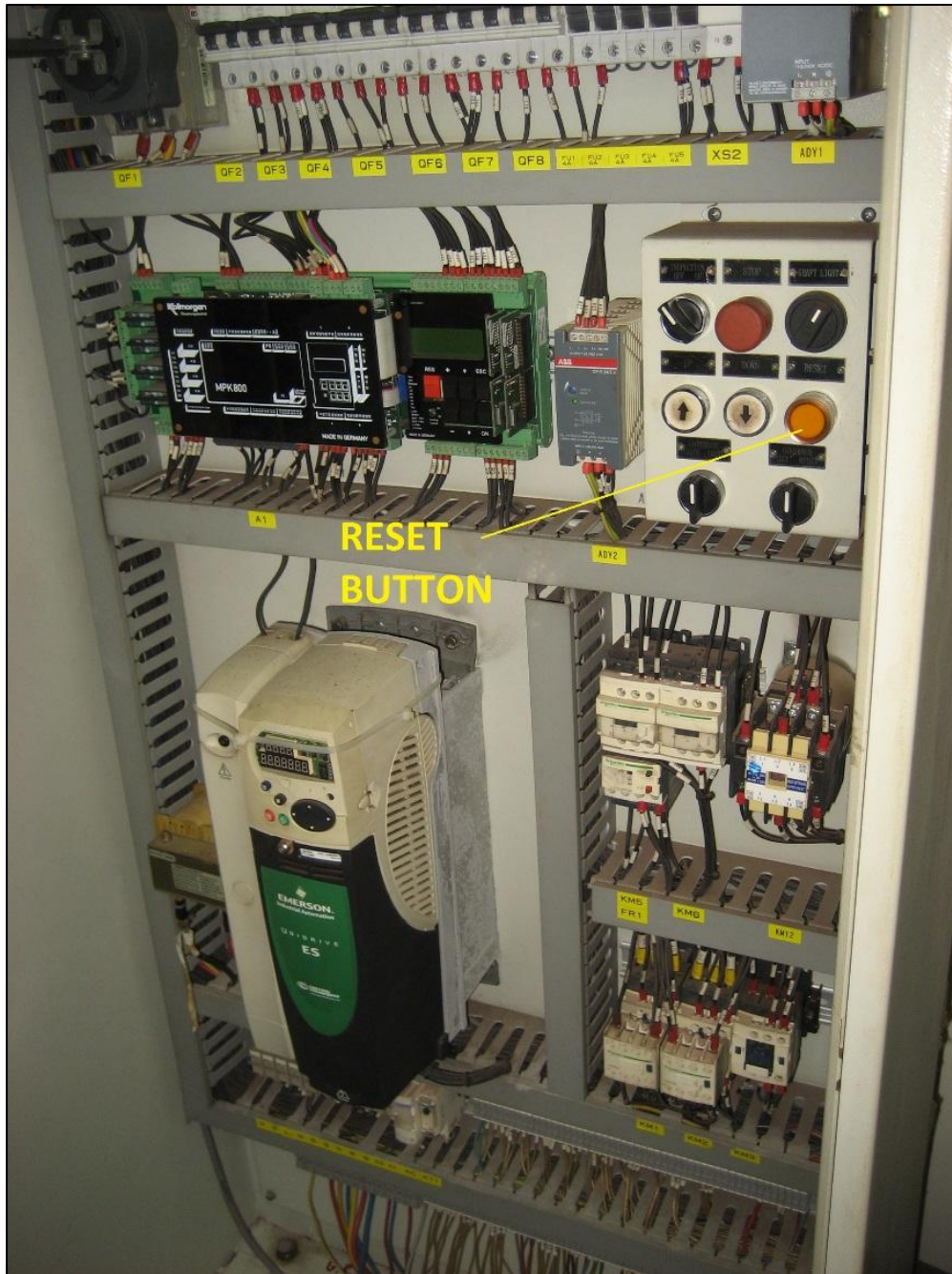
Figure 6: Reset button inside control cabinet
