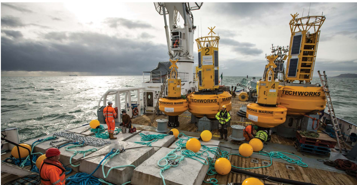
ILV Granuaile deploys Techworks Marine Environmental Monitoring Buoys - supporting Alexandra Basin Dublin Port re-development project Image credit: Techworks Marine
