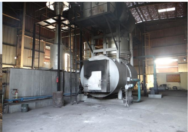
GMB TSDF_Incineration facilities (©C.Wohrer – 29.04.2016)
