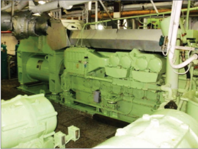
A diesel generator
