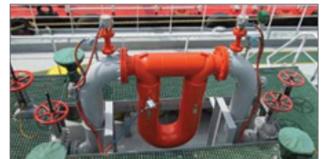
A mass flow meter installation
